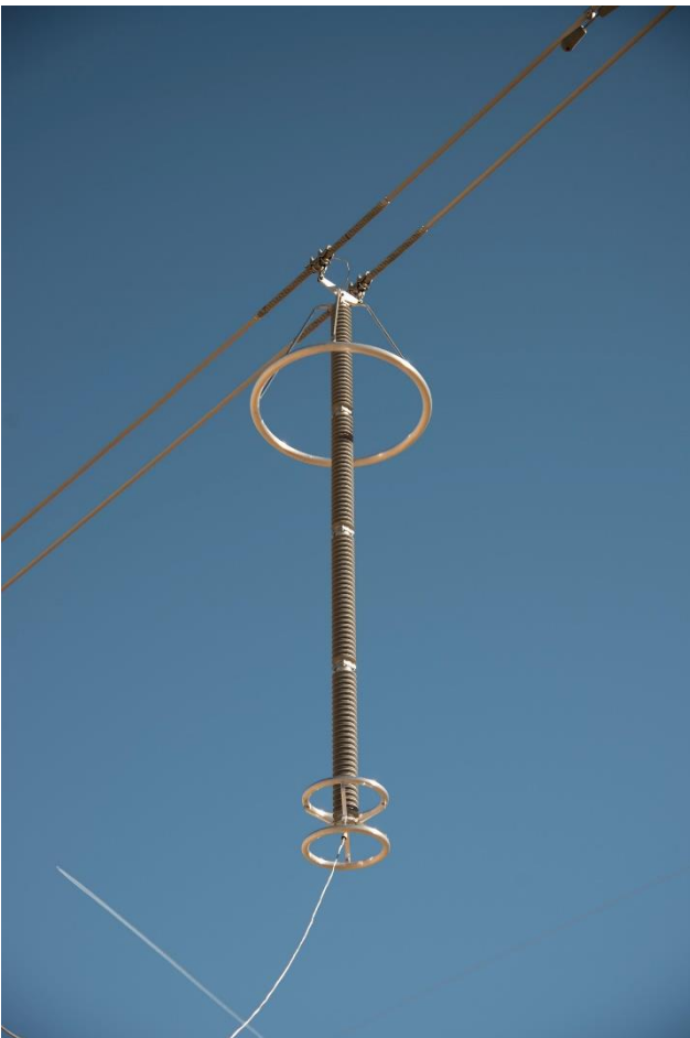
Non-gapped line arrester (NGLA)
